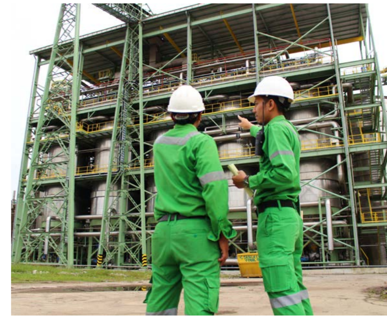
Equipment monitoring at digester
